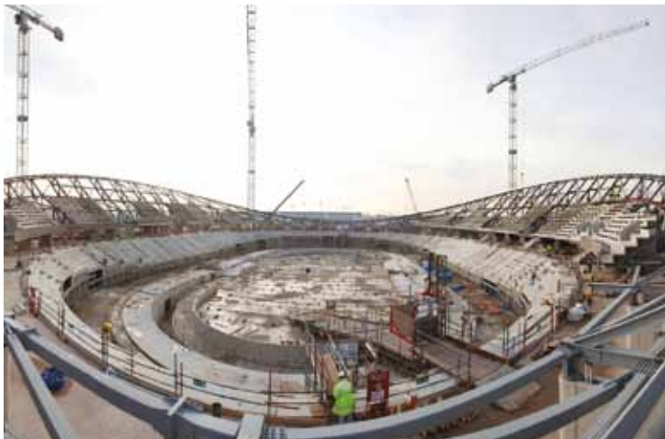
The steel structure, awaiting the roof, showing the twin ring beam – the ‘warped’ tennis racket frame – with the ‘rigid bowl’ of the 48 rib trusses which helps to transfer the tension from the cables down to the foundations © ODA
